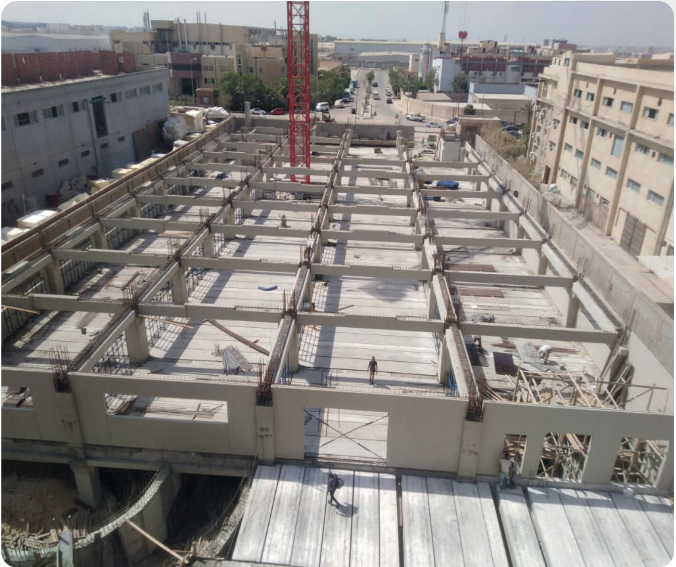
Large span with high loads floor to be covered by hollow core slabs ALsham factory - Obour City
