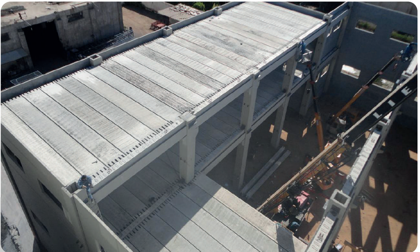
Minimum erection crew needed for hollow core slab Linetex factory - 10th of ramadan
