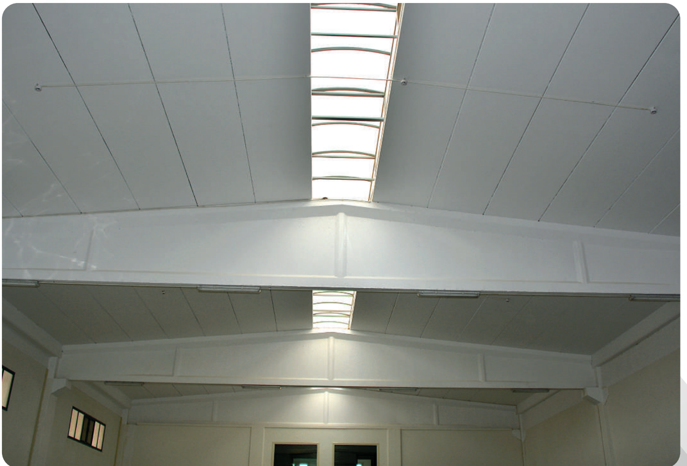
Hollow core slabs with paint finish & Skylight Line textile factory - 10th of ramadan
