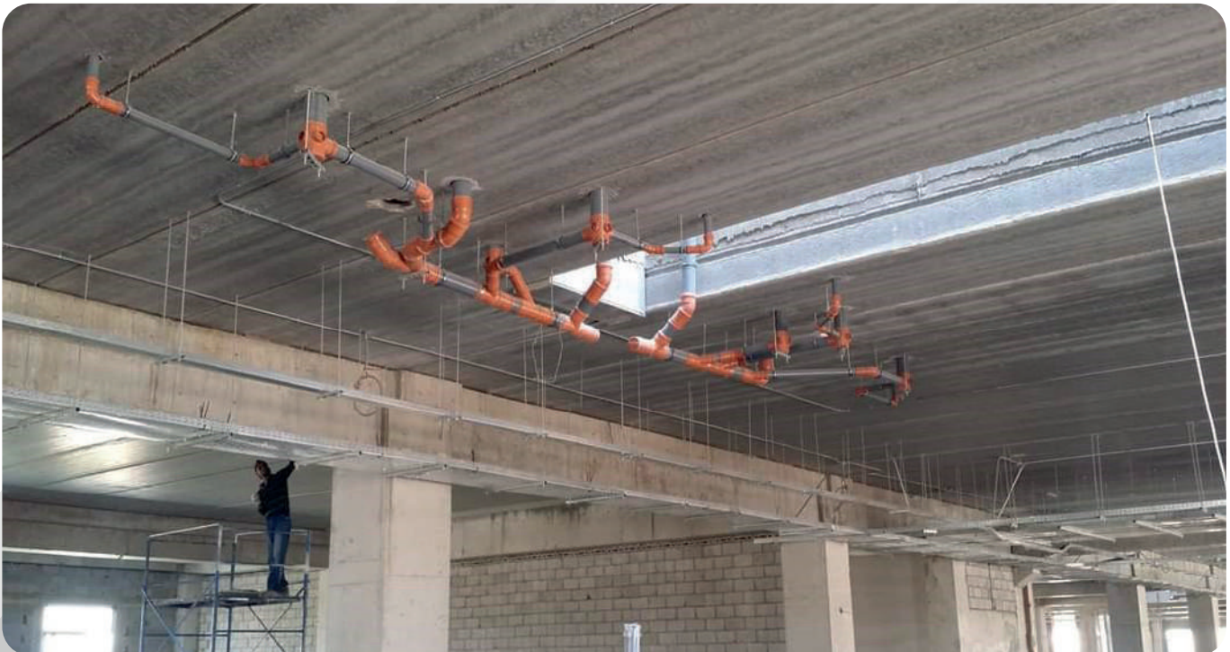
Cores in slabs used for extending pipes ORMAN school - 6 OCTOBER CITY
