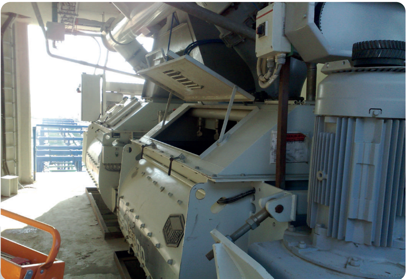
Double Automated concrete mixer
