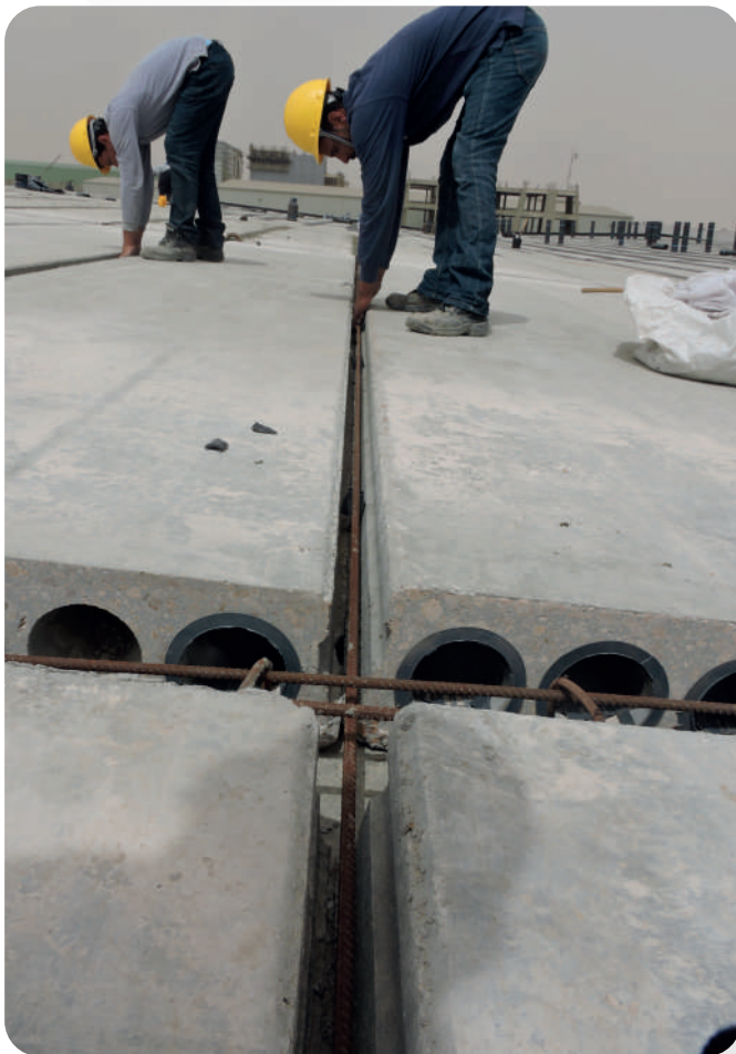
Preparing the joints for concrete filling Fourtex New weaving hall - Sadat City
