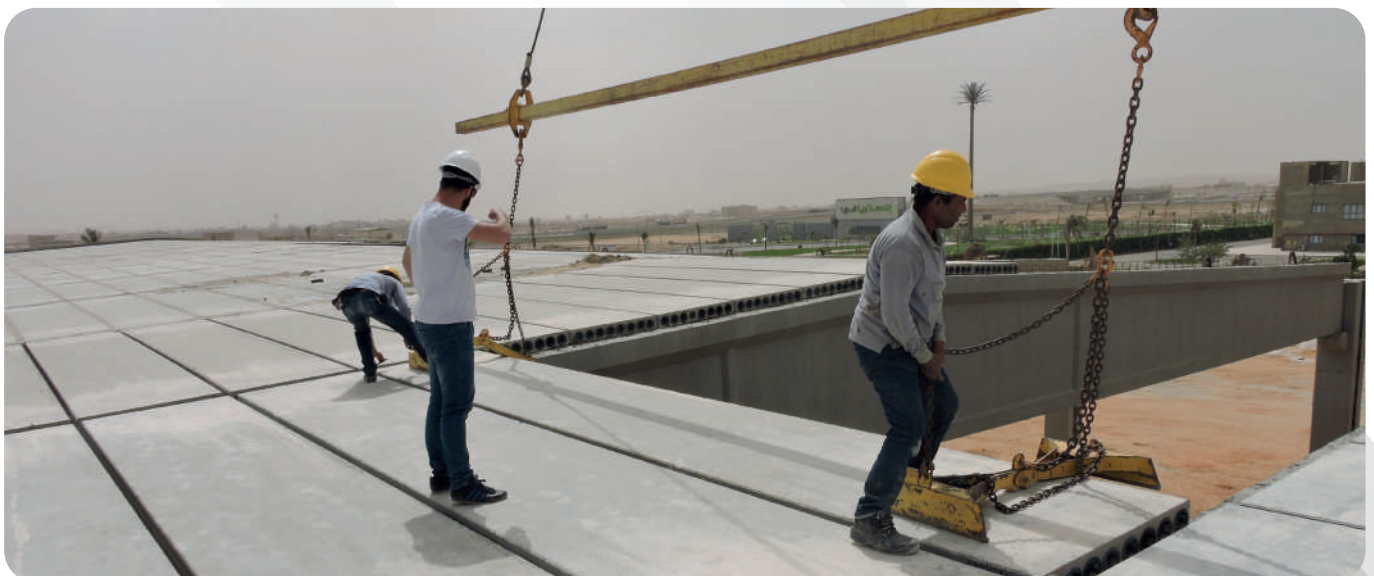
Hollow core slabs erection at required place BEDCO Textile factory - 10th of Ramadan
