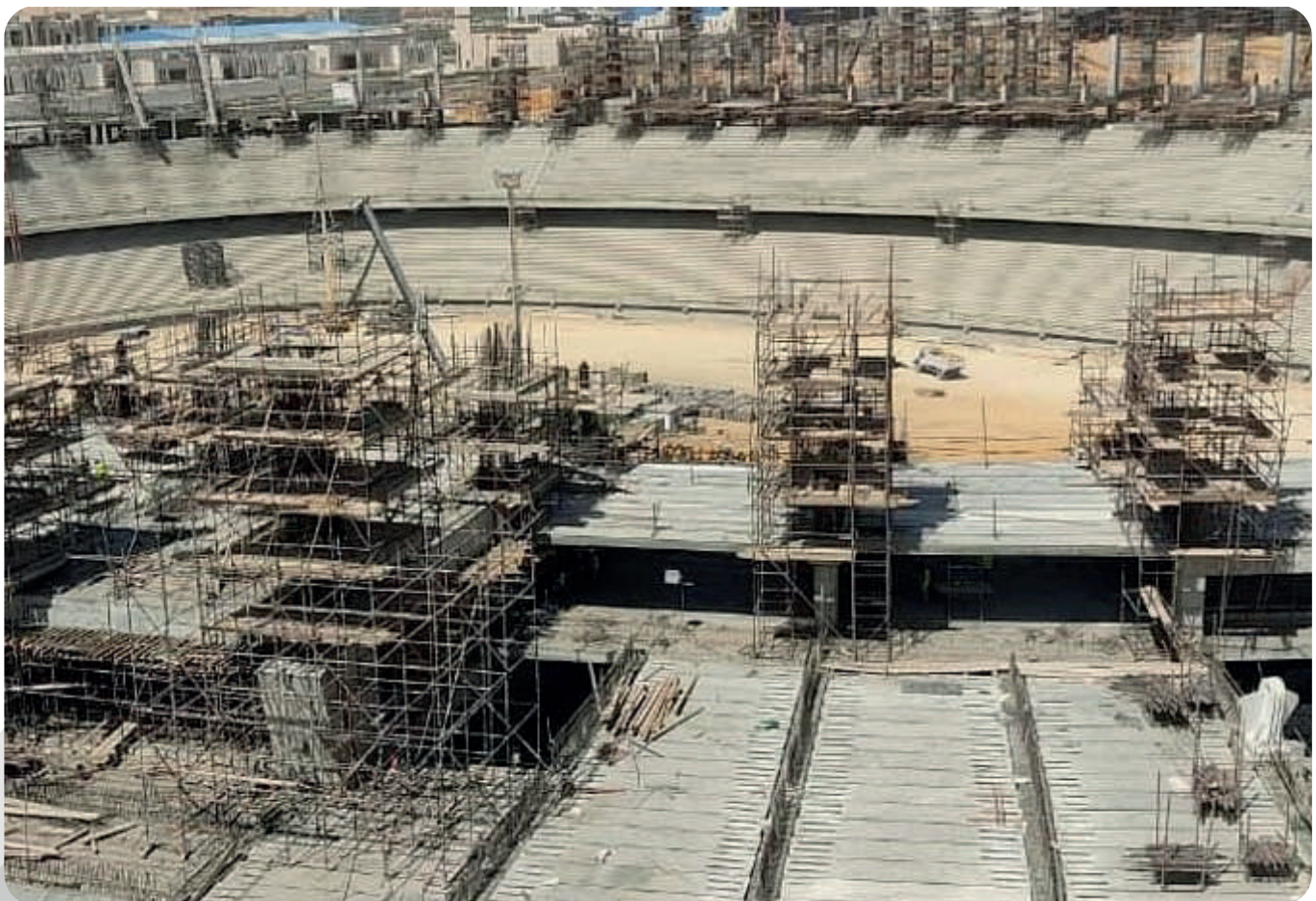
Hollow core slabs used in sports hall Olympic Stadium - Olympic Village
